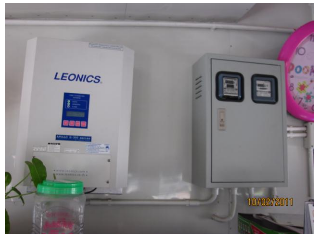
Figure 7. Grid connected inverter and energy meter.
