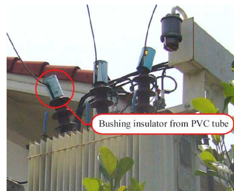
Fig. 2. Used of PVC water tube for protected a primary wire connection
