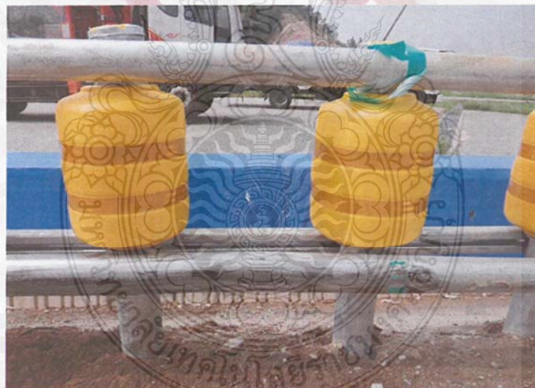
<Damage of Facilities After Car Collision>
