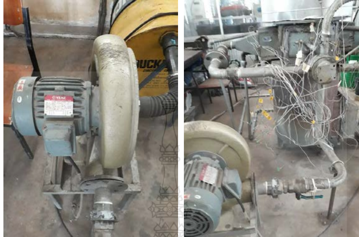
Figure 3.6 Air blowing system.
