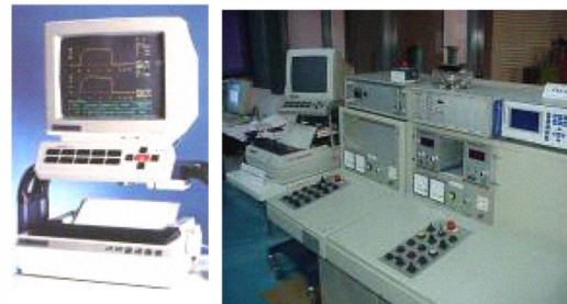
Fig. 13: Control and measurement devices
