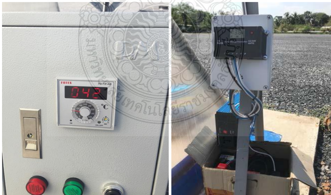
Figure 3-18 Photographs of equipment installation automatic temperature controller
