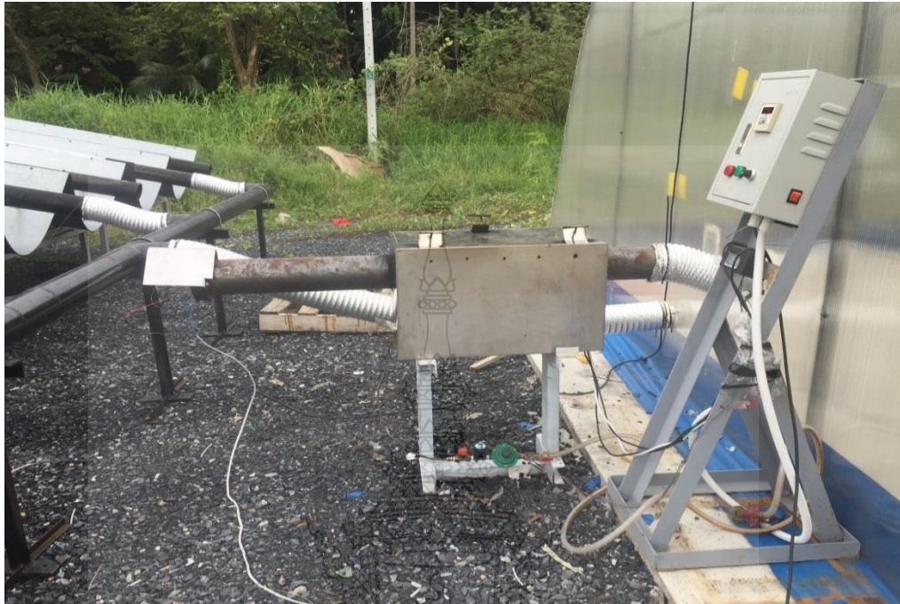
Figure 3-17: Photograph of installation gas burner
