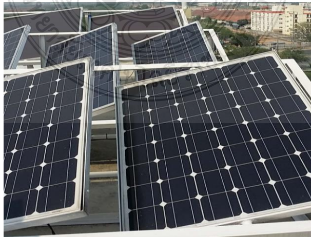
Figure 3.37 PV array installations at the PIER 93 building
