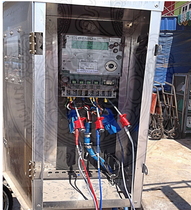
Figure 3.5 The connecting of the power quality analyzer at PCC.
