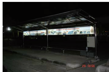
Fig. 1 PV bus stop system operated on night time.
