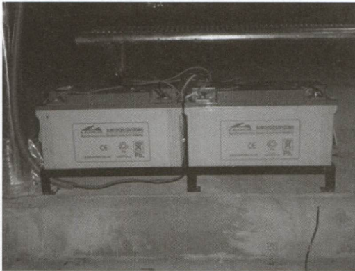
Figure 3 : Two batteries before conceal them within the compartment.
