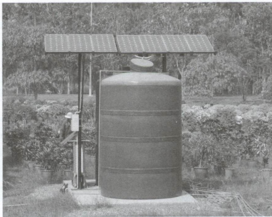
Figure 2: The PV water pumping system that seen from the south of the design location
