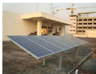
Fig 5 PV Grid Connected System used in this article
